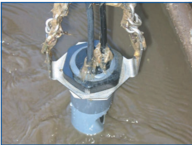
oxi::lyser in aeration tank
