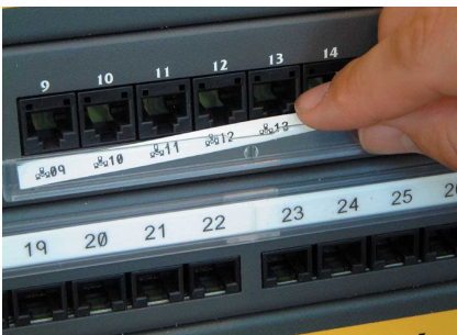
Punch block & patch panel labels
