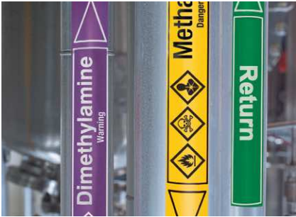
Pipe & valve marking
