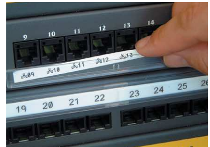
Punch block & patch panel labels
